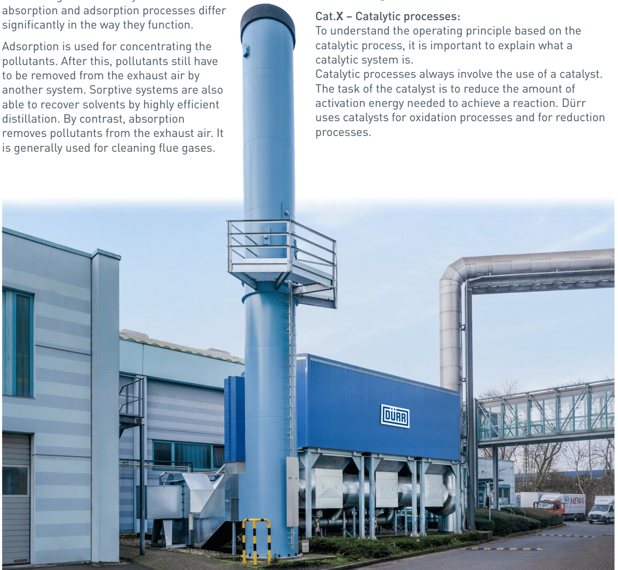
Picture 3: RTO technology for efficient air pollution control
